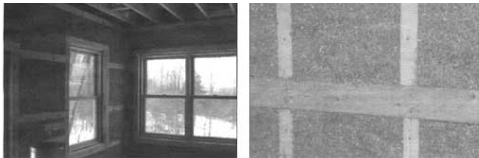
Figure 3 - The cellulose installers complained that the horizontal strapping interfered with the use of their rollers, making it hard to trim the cellulose flush (left). On his next house, builder Chuck Reiss packed out the studs with strips of rigid foam insulation, providing a surface to guide the trimming of the cellulose flush with the strapping. [Photo credit, both photos: Vermont Energy Star Homes]
