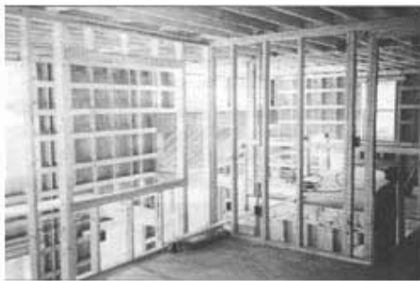
Figure 2 - Horizontal 2x4 strapping was used to reduce thermal bridging through the 2x6 studs. [Photo credit: Pat Hanson]
